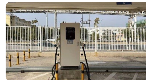
EV charging station
